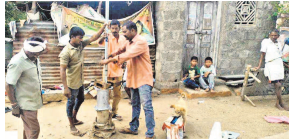
Scenes of people digging borewells and getting winding machines repaired have become common across villages in the State. (Above) A borewell being dug in Warangal.
